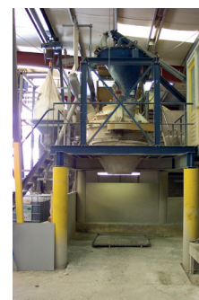
installation for the production of concrete.
